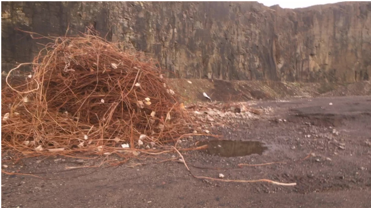
Above – some of the steel reinforcement, which was removed from demolition material, allowing ex demo concrete to be processing via Jaw Crusher.
